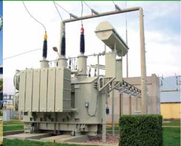
132/33kV Bangladesh Substation
