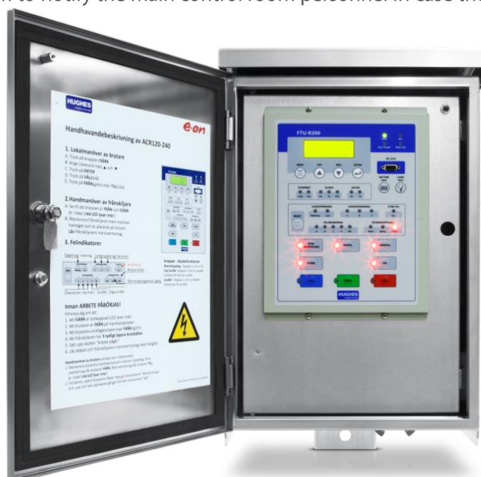
400x570mm stainless steel cabinet with FTU-R200 protection relay
